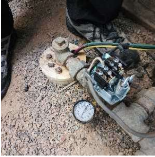
Well Head / Casing
